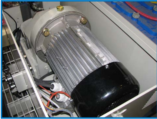
15 HP Electric Motor
