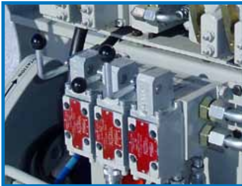
Low pressure valves for hydraulic make-up tool, rotation speed and hydraulic latching functions.
