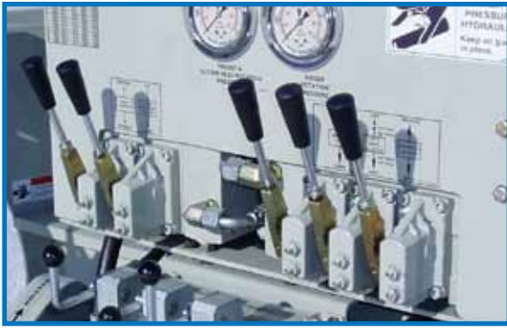
High pressure valves for jacking, rotation, frame travel, and PCH/PRH control functions.
