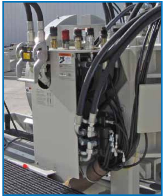
The quick couplers connect to the pressure, return, load sense, case drain hydraulic hoses from the GBM Power Pack, along with the PCH hydraulic hoses.
