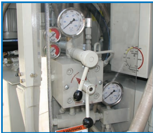
The dual ram & IJS control valve regulates the main jacking cylinders and the intermediate jacking station cylinders.
