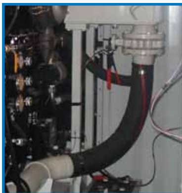
Suction Line Hydraulic Shutoffs With Integral Engine Starting Circuit
