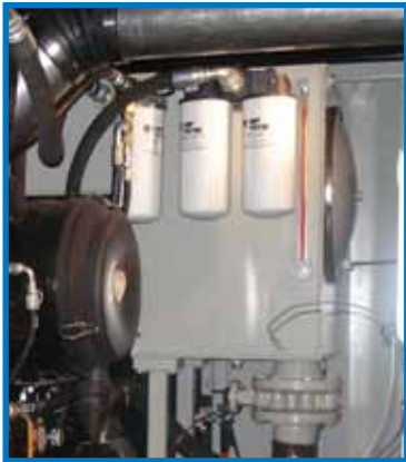
80 Gallon (303 L) Hydraulic Reservoir The hydraulic reservoir includes an oil level and oil temperature gauges.
