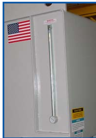
Hydraulic Reservoir Oil Level & Temperature Gauge
