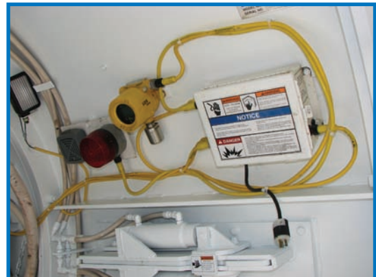
Methane Gas Detection System
