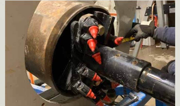
▲ The 18-inch cutter head featured retractable wing cutters that could be pulled back from the steel casing interior and a lead for the cutter bit to follow the pilot tube bore path.
