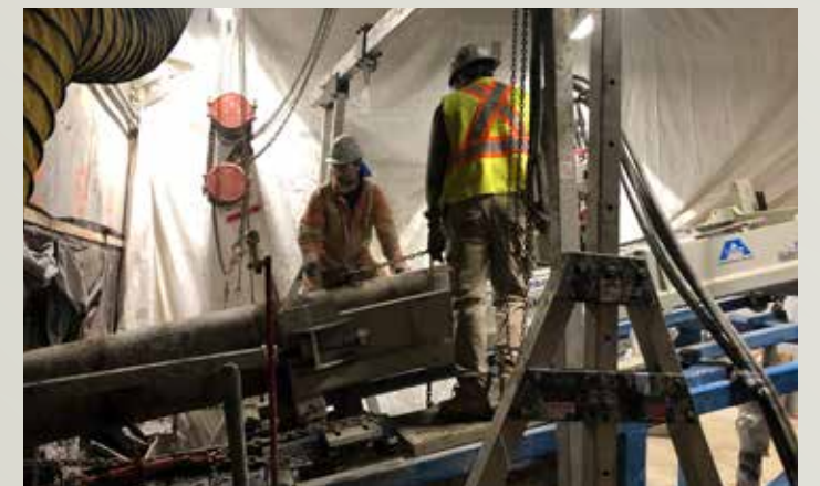
▲ The installation of 18-inch OD steel casing completed each bore, which will connect heating and cooling utilities to the new 25-story building.
