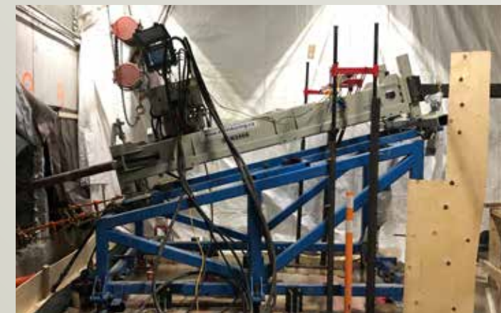
▲ EBCL's engineering team designed a specialized jacking frame stand to position the bore entry point to meet the design's line and grade requirements.
