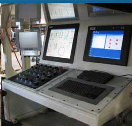
The control console car is where the operator monitors and adjusts all EPBM functions.
