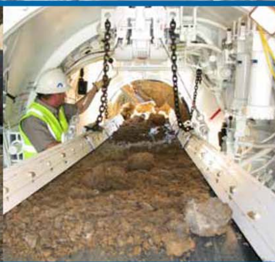
The operator's station is located along the inside of the TBM wall beside the conveyor. From this position, the operator can control the TBM steering and monitor or adjust as necessary.
