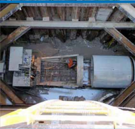
Shown here is a typical 5000 series in-shaft job site set-up.
