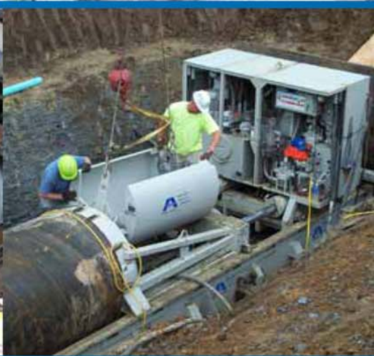
The outer ring of the thrust yoke provides a 360-degree surface to minimize point loading on the pipe. Contractors are returning the dirt bucket back to the haul unit after it has been emptied.
