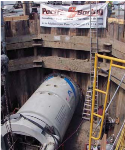
The 116-in. Akkerman EPBM will make way for 20-ft long sections of 96 ID tunnel pipe.
