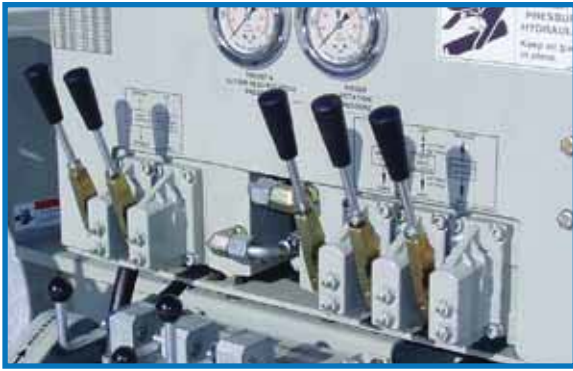
High pressure valves for jacking, rotation, frame travel, and PCH/PRH control functions.
