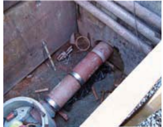
The final pipe string, installed accurately on line and grade, meets the concrete manhole where the rest of the shaft will be filled in and sealed off
