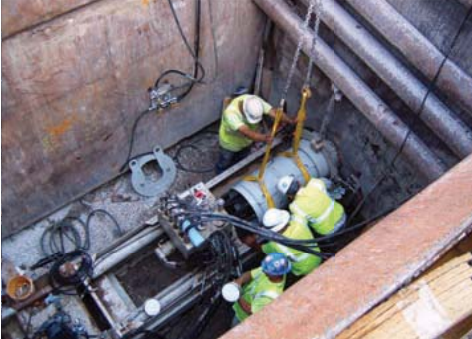
Crew members install the PCH on the GBM jacking frame after the casings and augers are installed
