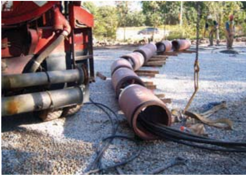
Above the jacking shaft, 1m segments of 400mm clay pipe are lined up and ready to be lowered
