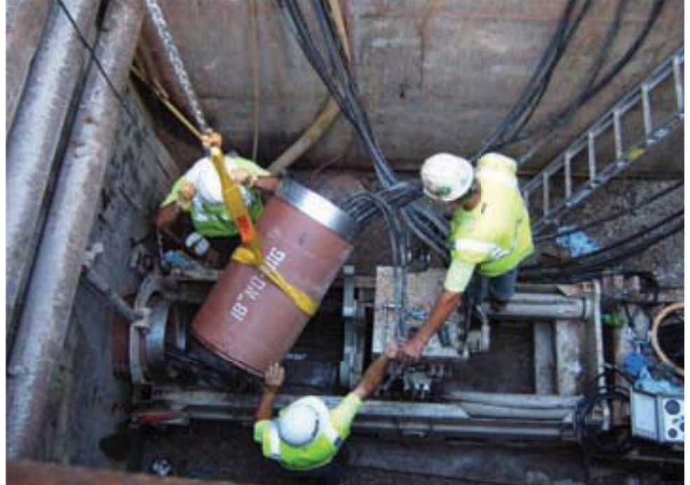
Bore Master workers install a section of vitrified clay pipe during one of five drives
