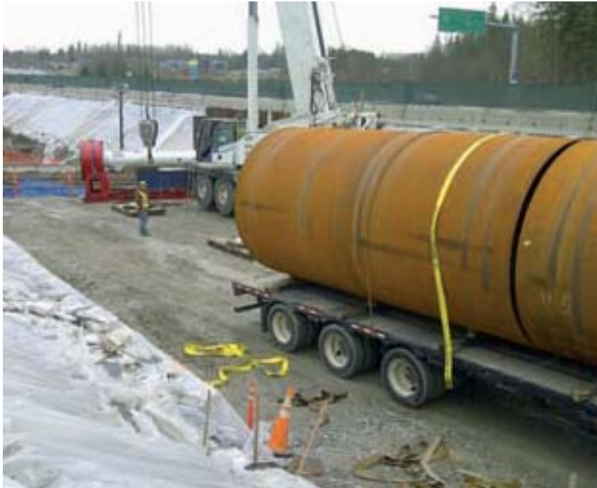
A crane lowers the HPD unit into the shaft and the 3m OD x 6m-long pipe for culvert installation arrives on site
