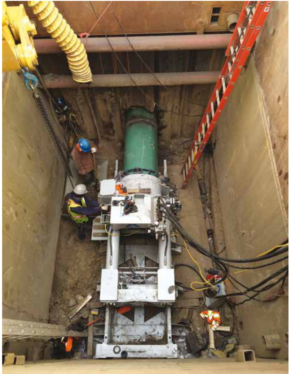
A range of 400 to 760-mm diameter gravity sewer laterals were installed under a pedestrian overpass at depths ranging from 7 to 10 m to avoid the area's many buried utilities.
