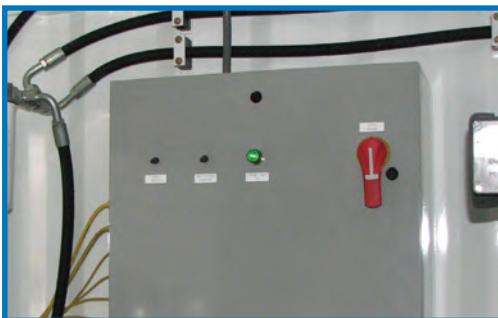
Electric Box with Main Disconnect Switch, Phase Error Indicator, Oil Cooler Fan Switch & Light Switch
