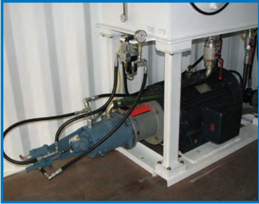
High Pressure Hydraulic Pump (13 gpm @ 8,000 psi) & 75 HP Electric Motor
