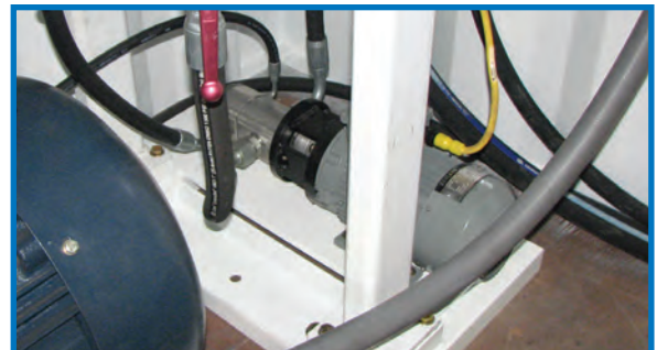
2 HP Electric Motor With Tandem Cooling and Pilot Pressure Pumps
