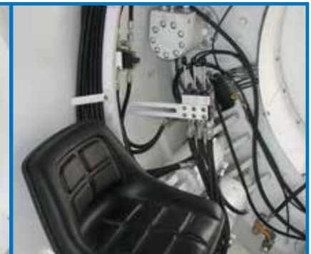
Operator station with pilot operated controls for the inner drum, conveyor, and auxiliary functions.
