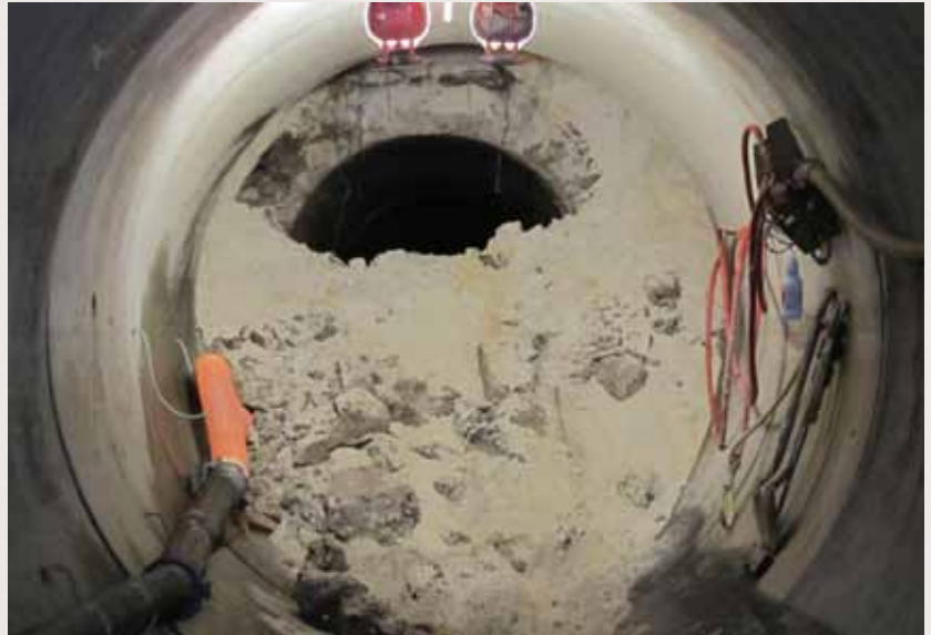
The photo, taken from inside the tunnel shows a pipe section meeting up with the original tunnel while excavated debris awaits removal.
