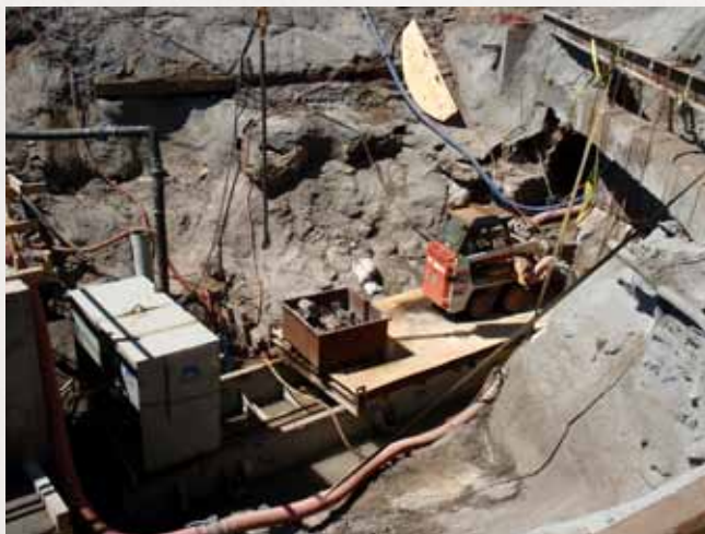
PCI Roads, LLC of St. Michael, MN used a 5000 Series Pump Unit, skid and thrust yoke to direct jack pipe as they increase the diameter of the 10th Avenue SE Tunnel in Minneapolis, originally hand mined in 1882.
