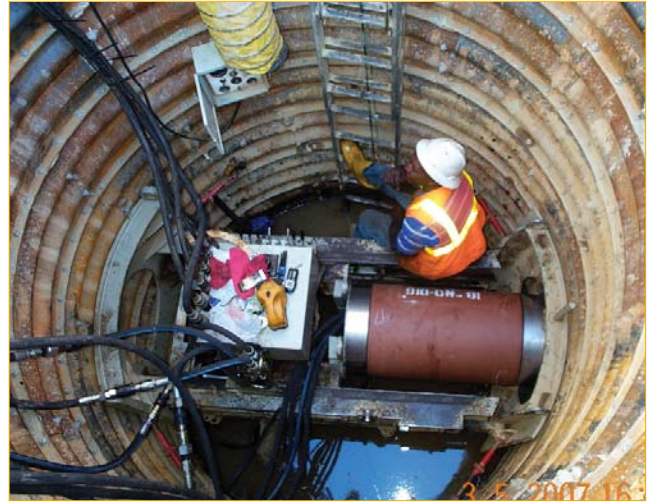
Workers were able to install 36 lengths of 1-m clay pipe — or a total of 118 ft in seven hours.
