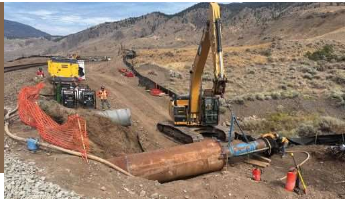
For the remote access project near Kamloops, British Columbia, Total Trenchless used two Grundoram Taurus pipe rammers from TT Technologies to install 12 casings of various diameters under an isolated rail line.
