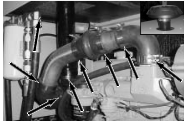
Air Intake System
