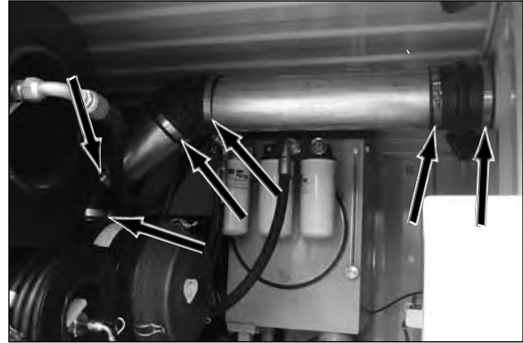
Air Intake System
