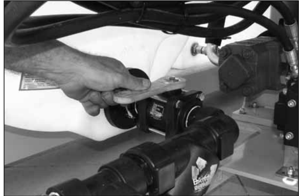
Jetting Tank Shut Off Valve Shown in Closed Position
