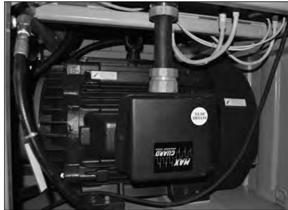
200 HP Electric Motor
