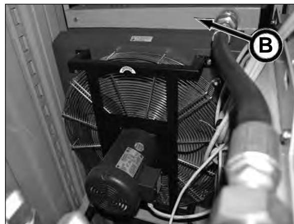
Oil Cooler Assembly Shown From Inside Container
