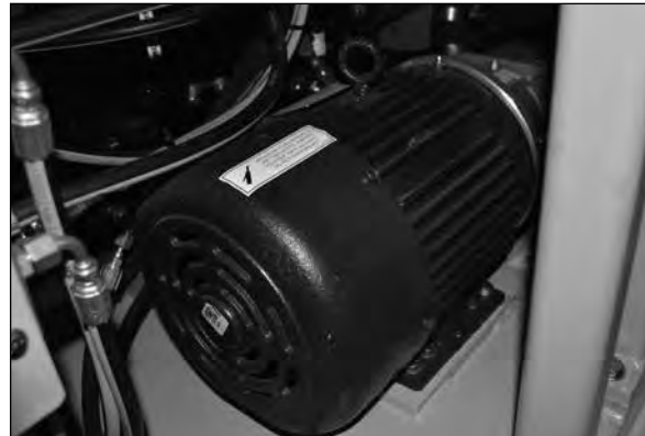
5 HP Electric Motor
