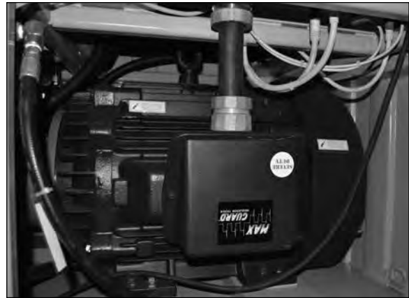
200 HP Electric Motor
