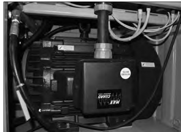
200 HP Electric Motor
