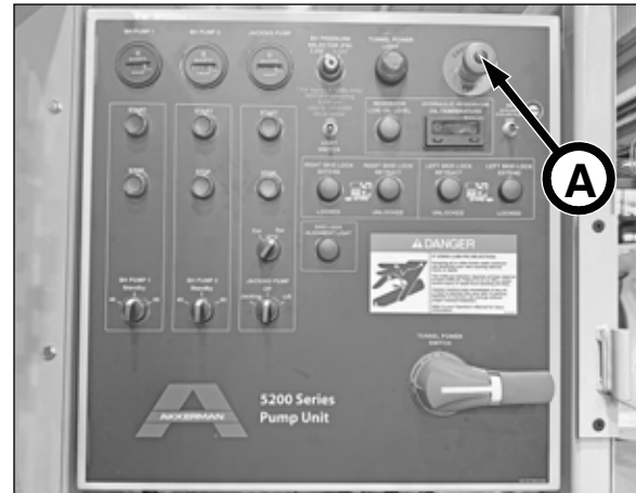
E-Stop on 5200 Series Pump Unit
