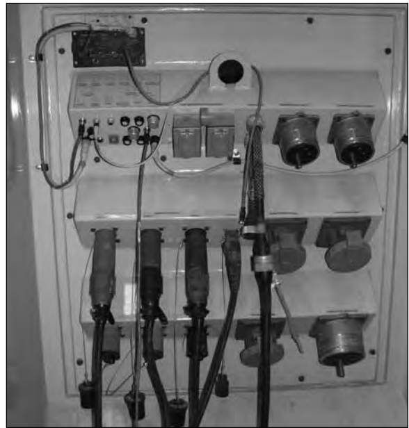
Control Container Bulkhead Connections
