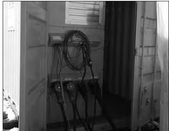
Control Container Bulkhead Connections
