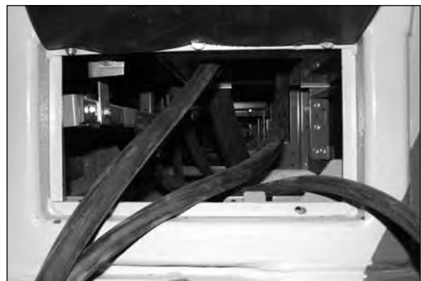
Control Container Power Lead Connections
