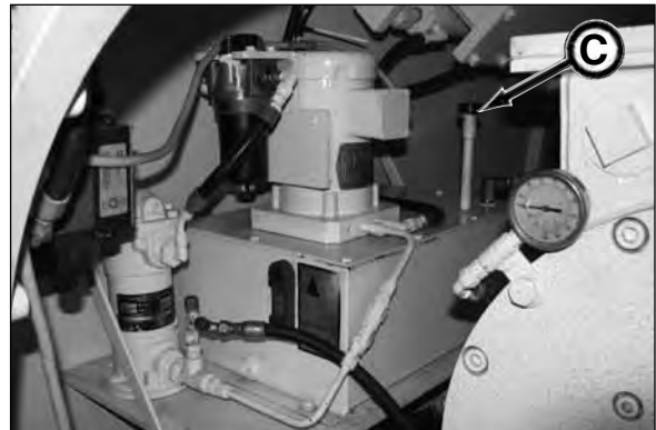
Oil Recirculating Pump MTBM Shown
