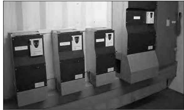
VFD Motor Controllers
