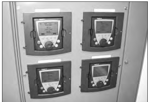
VFD Motor Monitors
