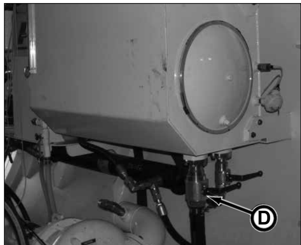
Main Hydraulic Shutoff Valve Shown in Closed Position Valve Must Be In Open Position Before Operating
