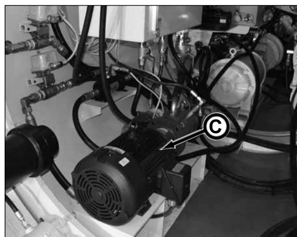
Lube/Jacking Can Main Hydraulic Motor
