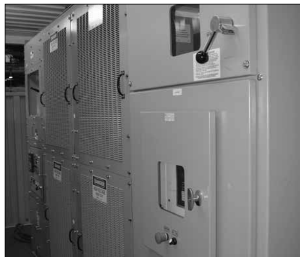
Main Drive Power Container (SN FA22062F)
