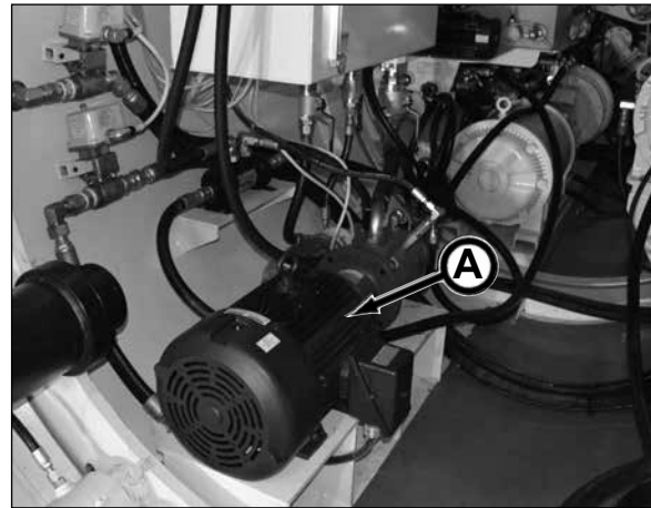
Lube/Jacking Can Main Hydraulic Motor
