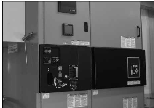
Main Drive Power Container (SN FA22080F)
