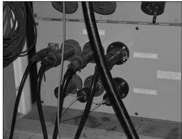
Control Container Bulkhead Connections
