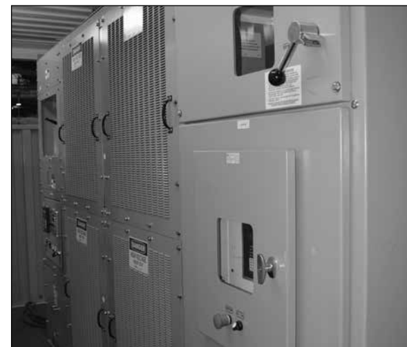
Main Drive Power Container (SN FA22062F)
