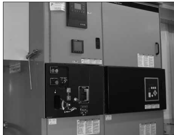
Main Drive Power Container (SN FA22080F)
