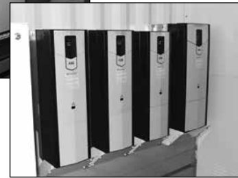
VFD Motor Controllers
