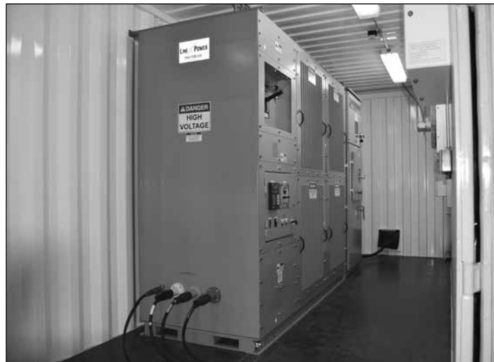
Akkerman Main Drive Power Container
