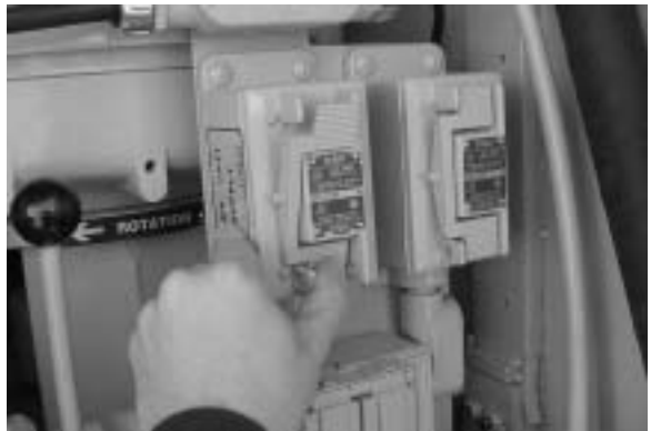
Pump Unit Power Supply OFF
