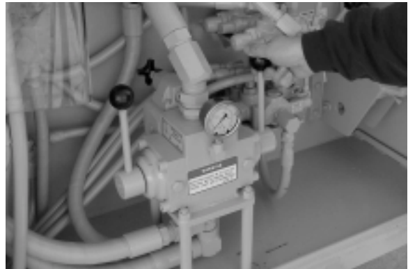
Auxiliary Pump Unit Dual Valve Volume OFF
