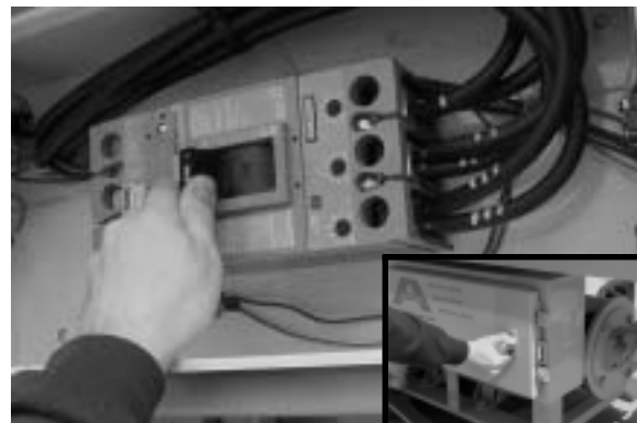
Disconnect Switch Shown In ON Position
