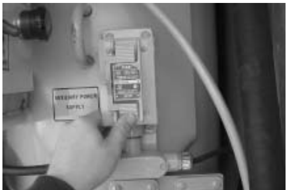
Auxiliary Power Supply OFF
