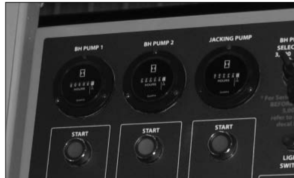
5200 Pump Unit Hourmeters
