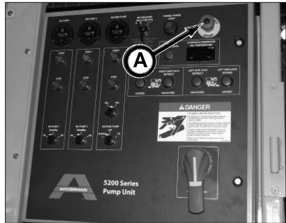
E-Stop on 5200 Pump Unit
