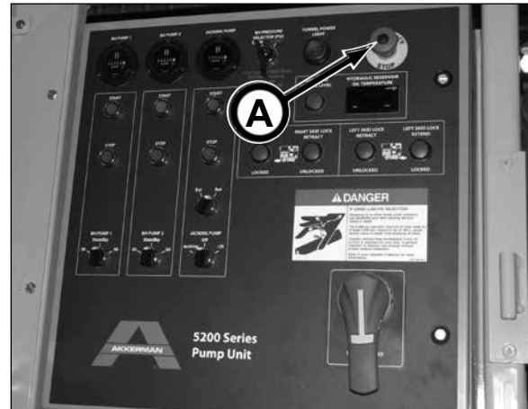
E-Stop on 5200 Series Pump Unit
