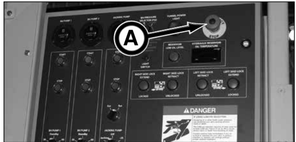
E-Stop on 5200 Series Pump Unit
