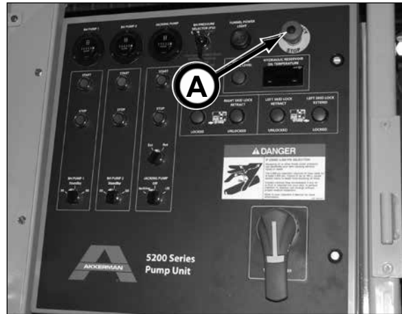
E-Stop on 5200 Series Pump Unit
