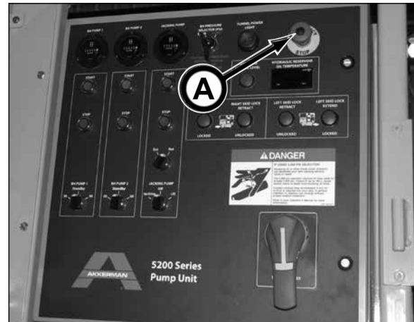
E-Stop on 5200 Series Pump Unit
