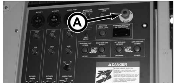
E-Stop on 5200 Series Pump Unit
