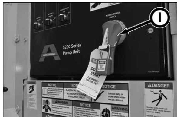
Tunnel Power Switch on 5200 Pump Unit Control Panel in LOTO
