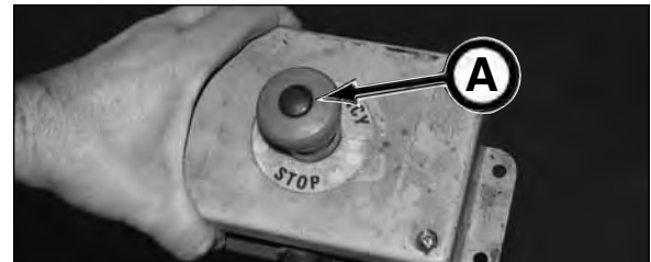
Remote E-Stop on 5000 Series II Pump Unit
