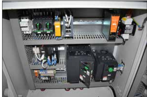
Foam electrical box terminal blocks shown
