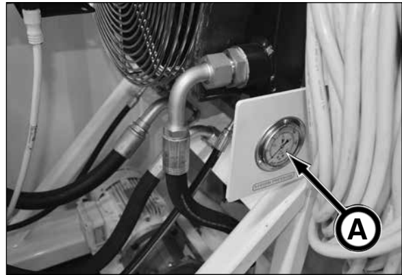
Hydraulic Power Pack System Pressure
