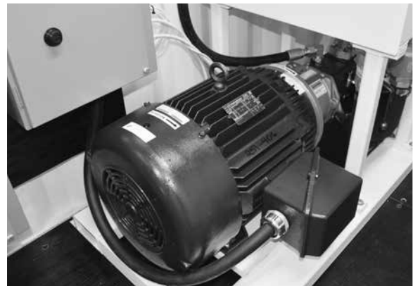
50 HP Electric Motor
