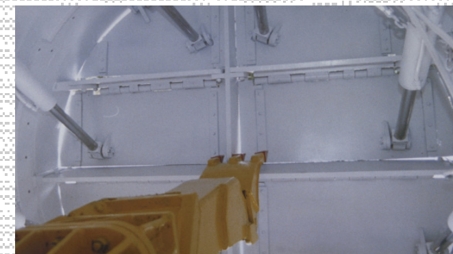
Figure 7. EBS equipped with hydraulic closeable doors to prevent subsidence.
