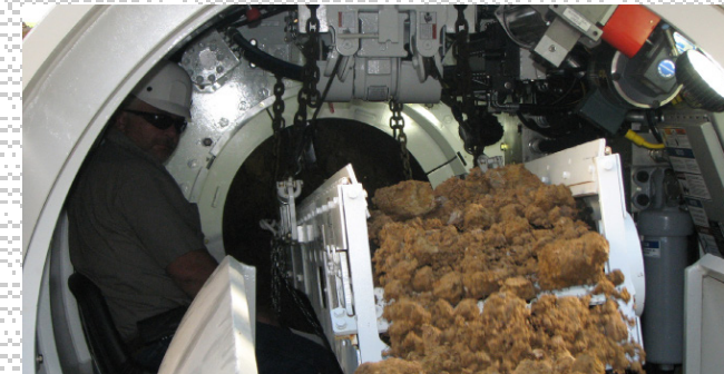
Figure 2. The operator's control station is located inside the TBM alongside the spoil removal conveyor.
