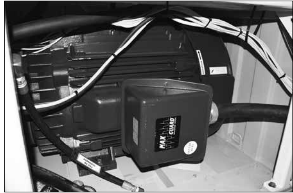
166 HP Electric Motor
