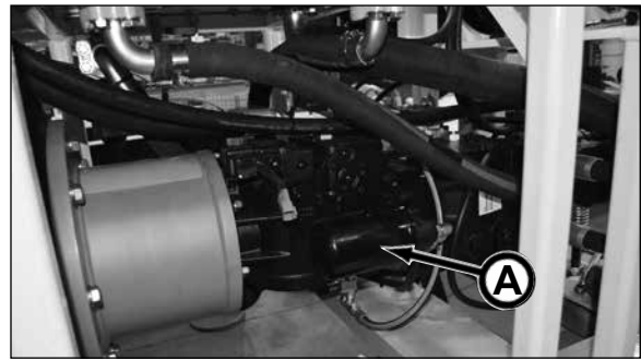
Drive 1 Pump Filter
